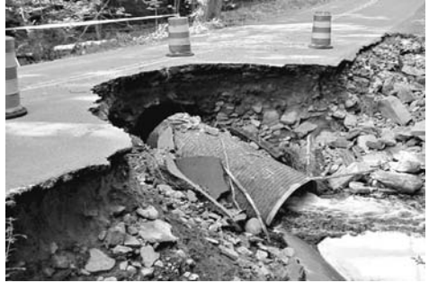
Stormwater damage to community infrastructure
